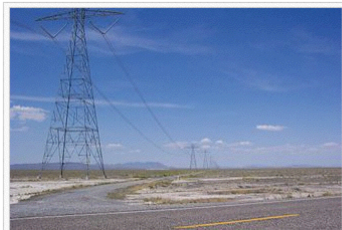
The Intermountain HVDC power line. Picture taken in Utah along U.S. Route 50
