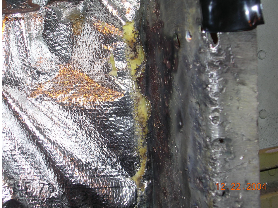
Figure 7. Low current damage to blanket.
