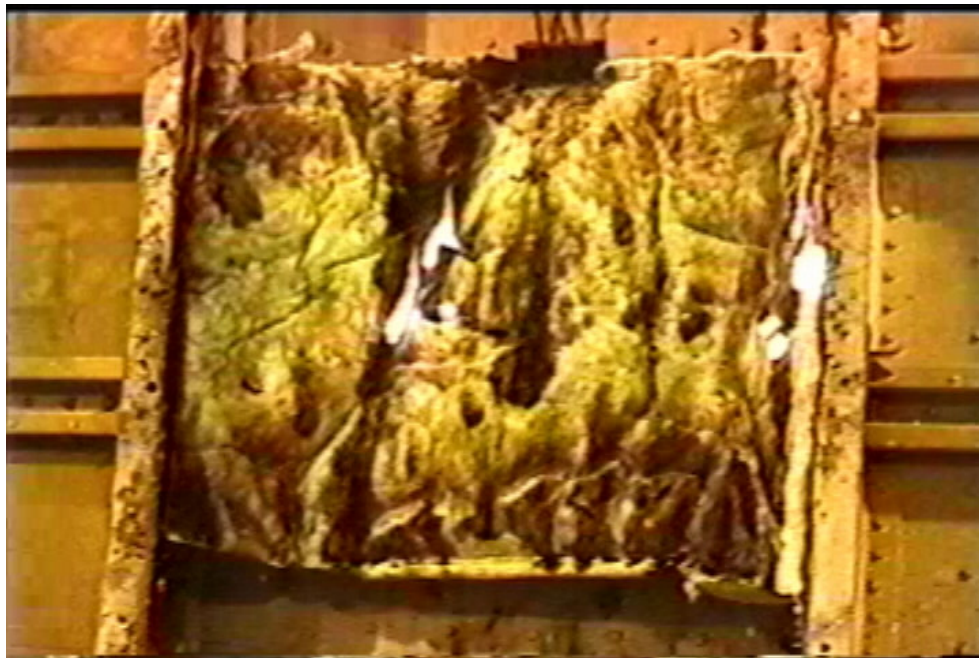
Figure 4. Plain Mylar™ 0.6 PCF Arc Damage (front side film totally consumed).
